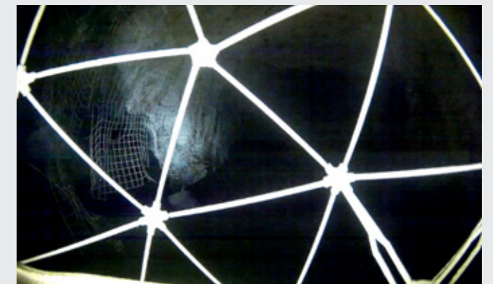
UNSUPPORTED GROUND IN A NO-GO ZONE
